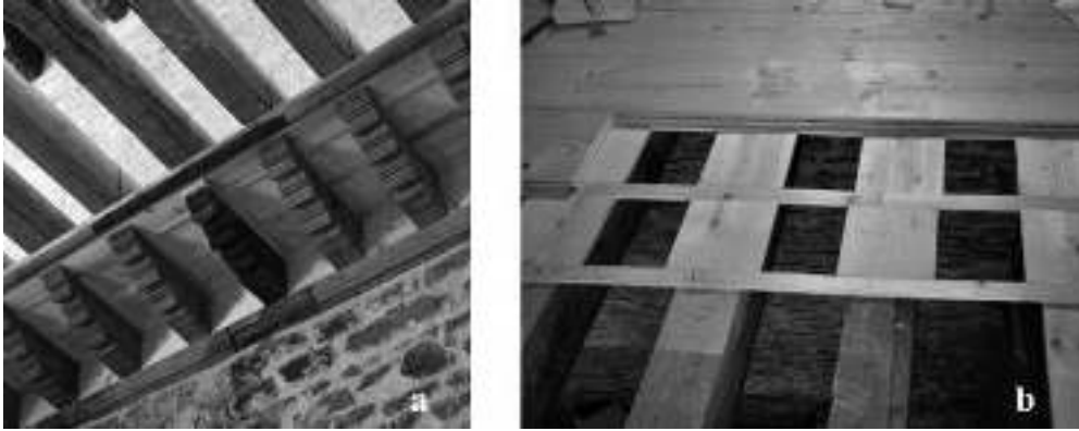
Figure 10. a. The in situ remaining original 12 th corbel and underlying cornice, with the new corbels and beams. The lower coffered ceiling between corbels and beams is already in place. Discernible is the original braid element, that was found reused in the Ottoman wing by chance. b. Constructing the coffered ceiling over the beams. The cantinelle running transversally to the beams are made of strips as original, whereas the ones parallel to the beams are made of planks projecting over the edges of the beams, ensuring full contact of floor boarding and beams. Note some tongue and groove boarding planks that have already been screwed into place
