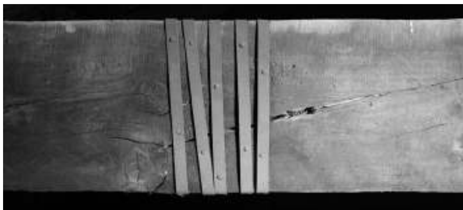
Figure 8: System used for the strengthening of the tie-beam of truss 5 (photo by E. Zamperini).
