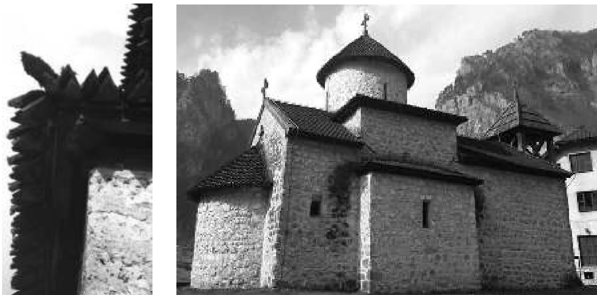
Figure 8: Details of roof cladding decay and rain water traces on walls of Monastery Dobrilovina
