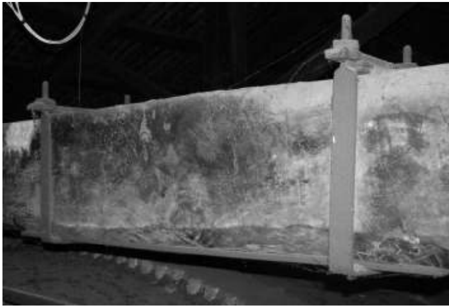
Figure 9: System used for the strengthening of the tie-beams of truss 2 and 4 (photo by E. Zamperini).
