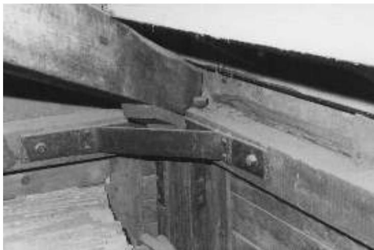
Figure 10: Metallic handmade elements to stiff and reinforce angle beams in the upper part of the structure. San Sperato House (Reggio Calabria); similiar to the one of Cav. Ferruccio Gay at the beginning of ‘900.
