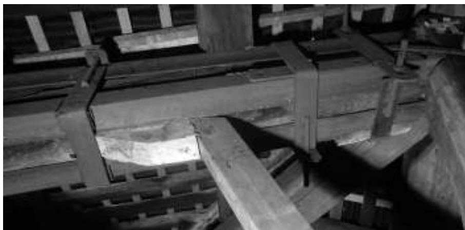
Figure 14: Strengthening system for the rafter of truss 5 (photo by M. Bosi, A. Cernuschi, E. Doria, P. Pilan).
