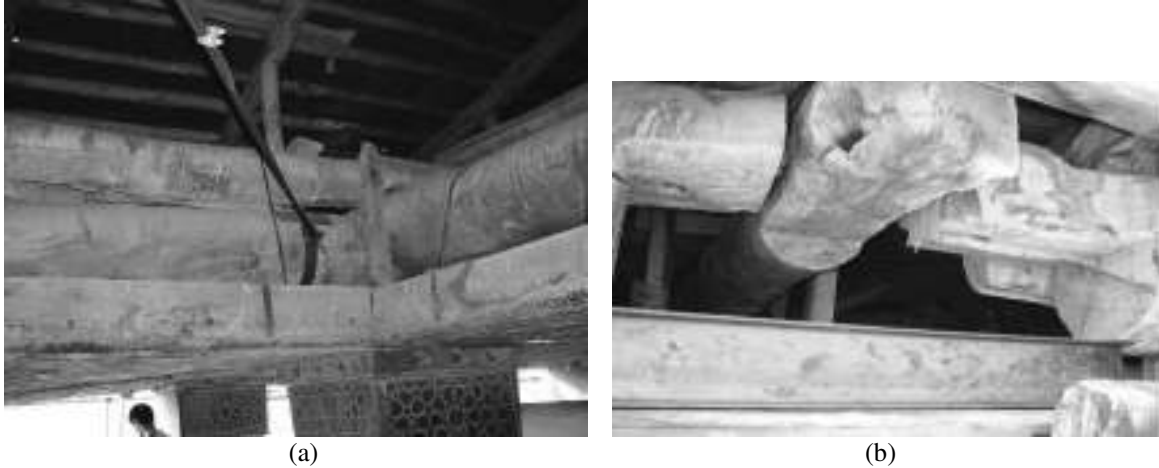
Figure 17: (a) Secondary beam over the main beam over the column with a steel cable lateral bracing attached to the main beam, (b) a steel profile for strengthening the wooden beam
