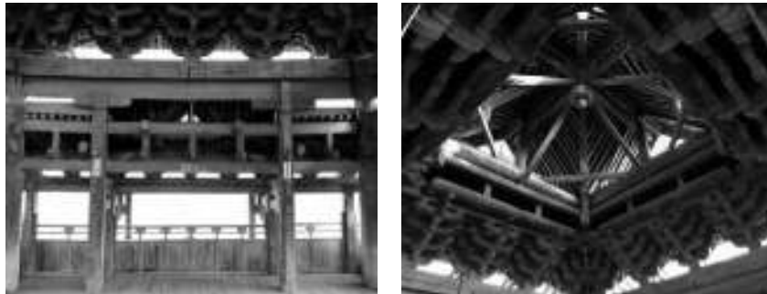
Figure 5: The columns, girders of the third floor and the bracket set on the top of Feiyun Pavilion
