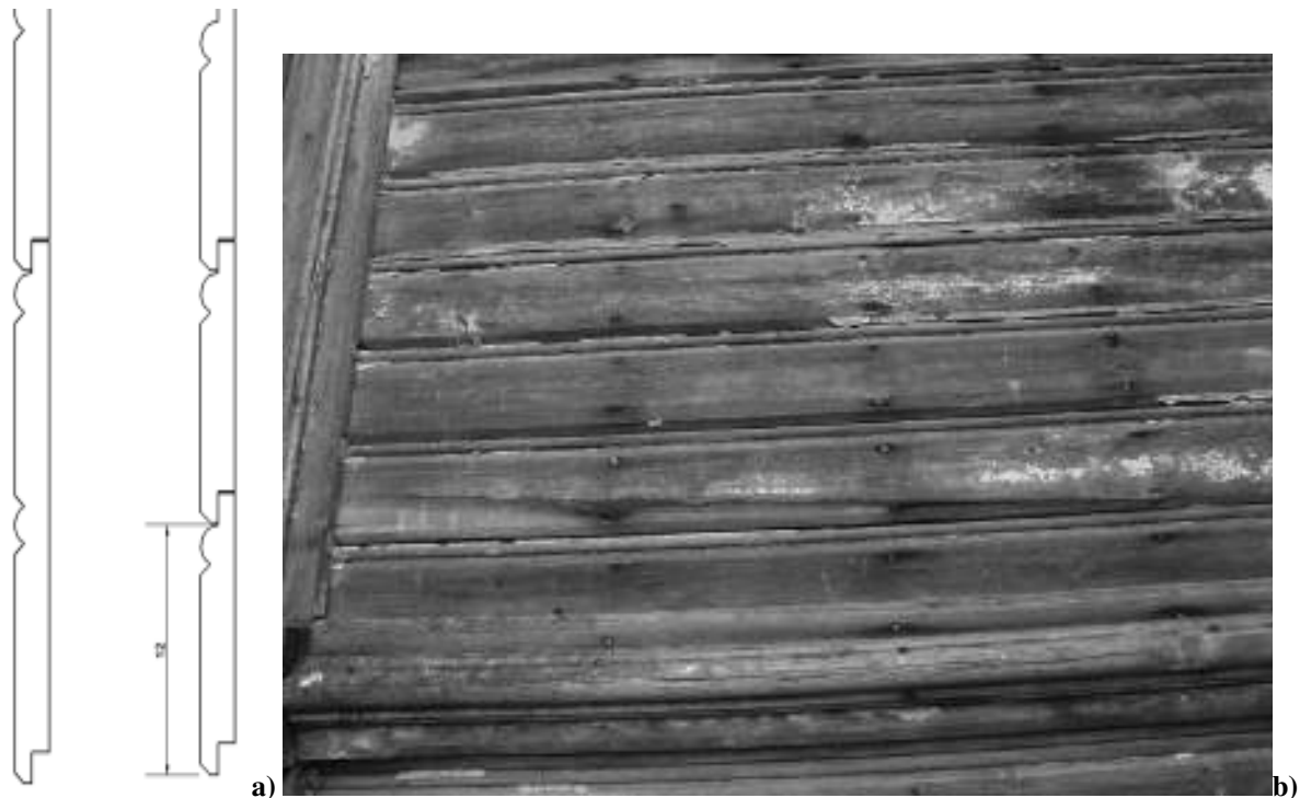
Figure 4. Machine shaped boards a) drawing and b) façade of a house at Prinkipo Island, Istanbul (Drawing and Photo: D. Acar)
