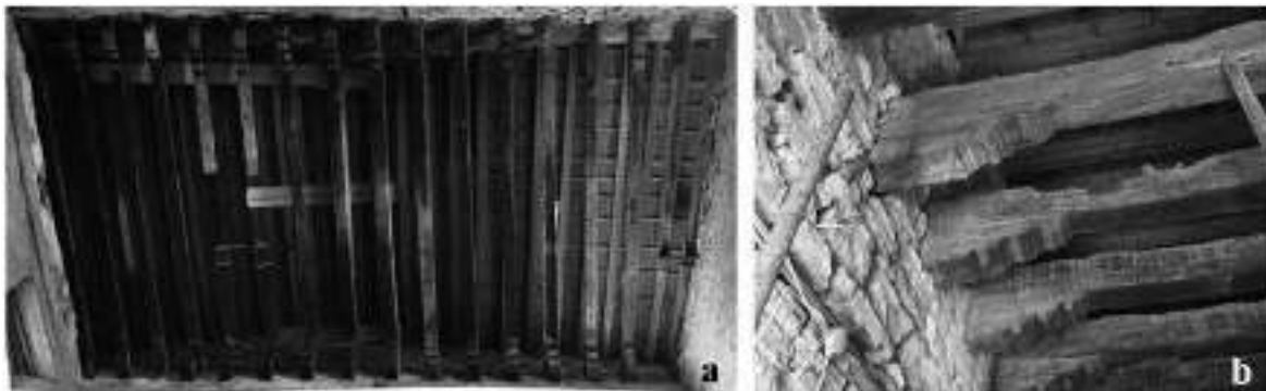
Figure 5. a. The second floor remains, underneath the modern roof. b. Closeup of some of the second-floor beams and corbels, before restoration began
