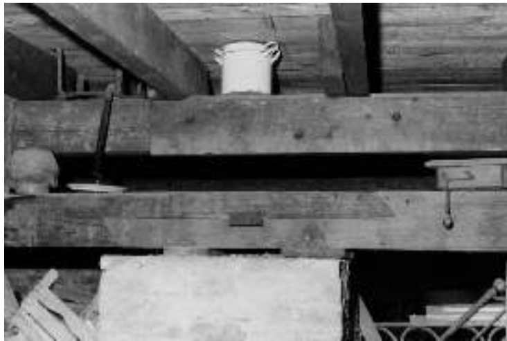
Figure 9: “stop-splayed scarf with key” joint that connect two sleeper in the foundation. San Sperato House (Reggio Calabria); similar to the one of Cav. Ferruccio Gay at the beginning of ‘900.
