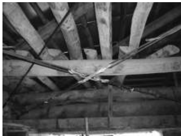
Figure 18: Wooden horizontal bracing system replaced by a steel cable bracing system that is too stiff
