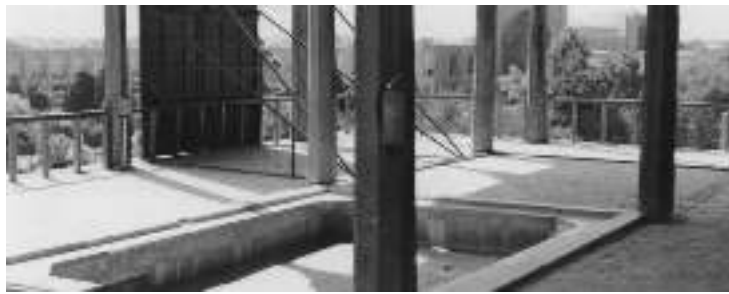
Figure 21: Inadequate fire distinguishing system, Ali Qapu building, Isfahan, 1597-1668 A.D.
