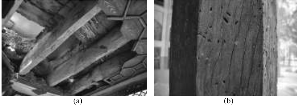
Figure 20: (a) Termite attack, Mosavver-al-Mulki house, Isfahan, eighteenth century A.D., (b) beetle holes, Hasht-Behesht building, Isfahan, 1897 A.D.
