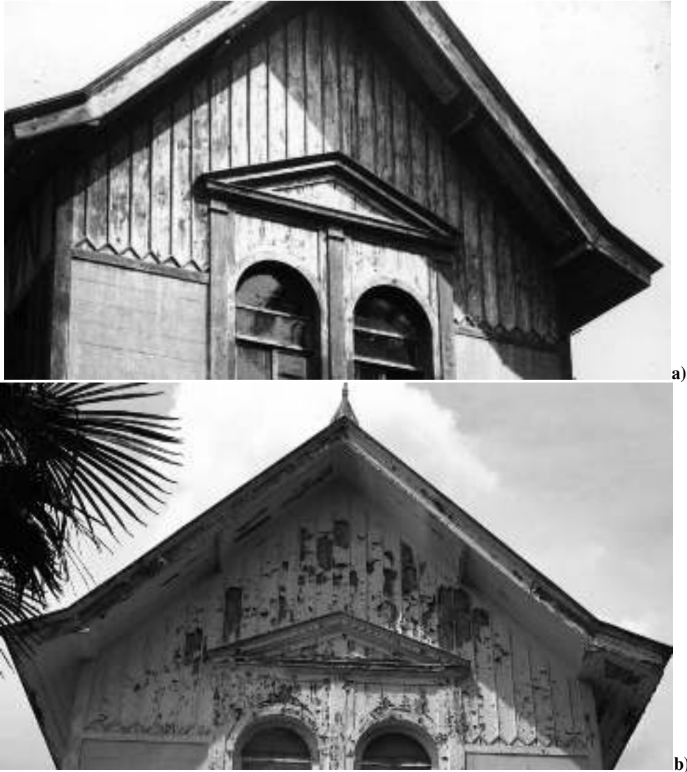
Figure 6: Roof forefront of Prince Kemaleddin's house in Dolmabahçe Palace showing the aging of a) linseed oil paint (1966 – Turkish National Palaces Archive) and b) modern plastic paint (2008 – D.Acar)
