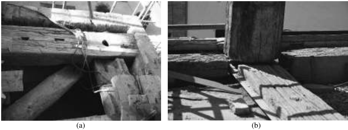
Figure 13: Floor ties between the columns: (a) corner, (b) strengthened with steel profiles
