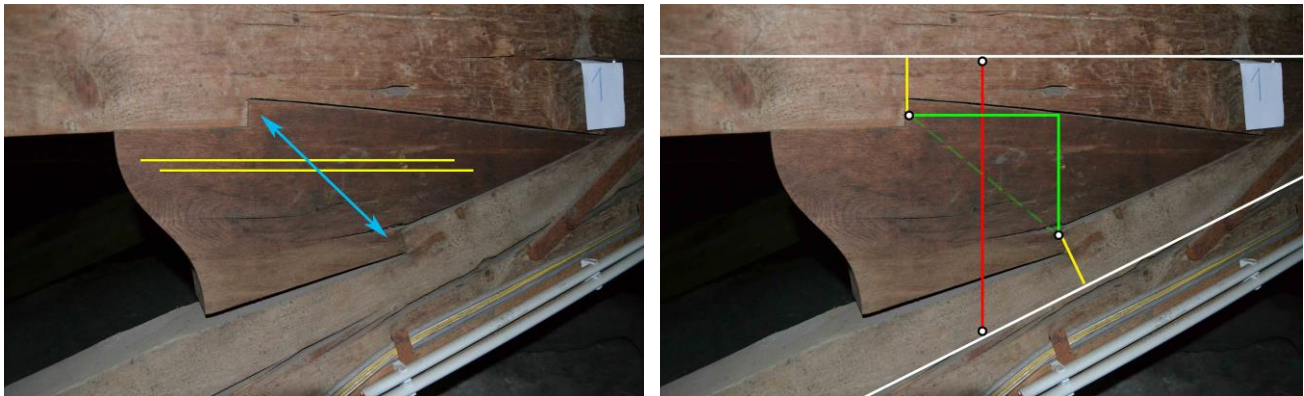
(a) Triangular block of oak: Grain direction (yellow) and compressive force (blue)
