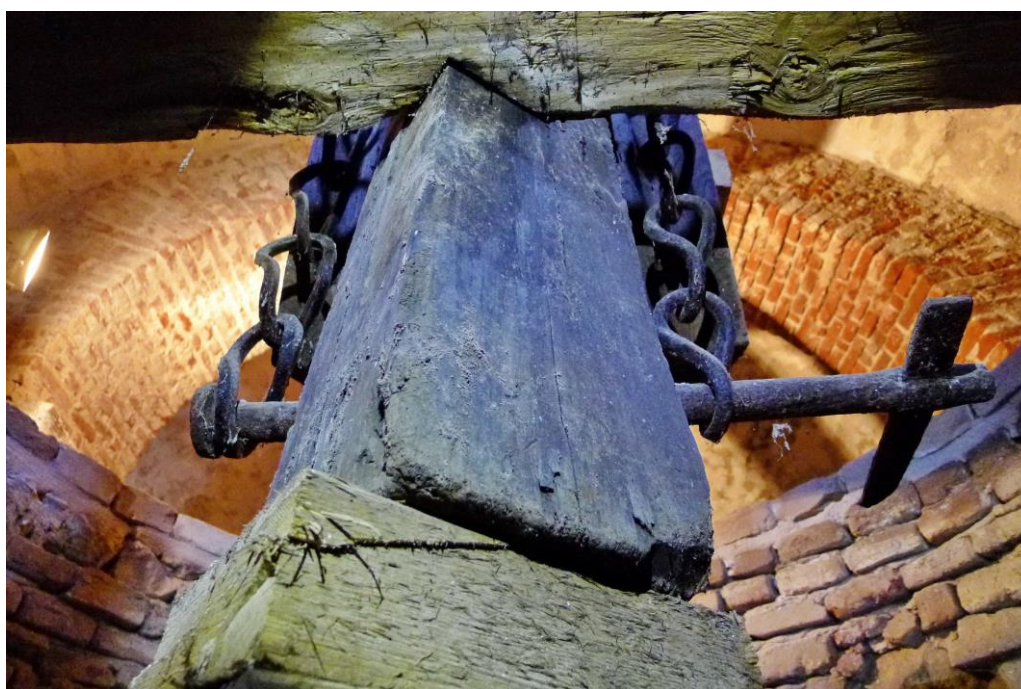
Figure 5: Bottom view of hinge at the lower end of the main post guided by the notch in the transverse beam, photo Jiří Bláha, 2015.
