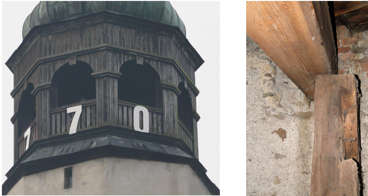
Figure 1: Lower lantern of the tower (left). Element connecting the structure of the lantern with the masonry core of the tower (right)
