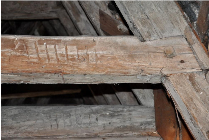
Fig. 6. Toruń, 6 Mostowa Street. Roof structure of building B. The connection of the rafter with a collar by means of a single dovetail lap joint (Photo by U. Schaaf).
