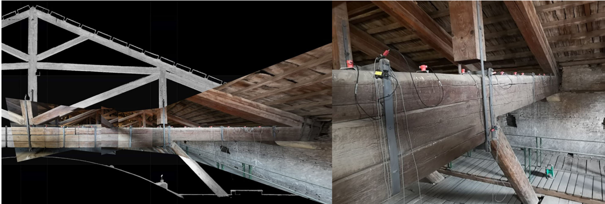
Figure 3: One of the 18 inspected timber trusses of the San Pietro cathedral in Bologna. Placement of vertically polarized geophones connected to a SoilSpy digitizing system. @Prati, Isani, 2019
