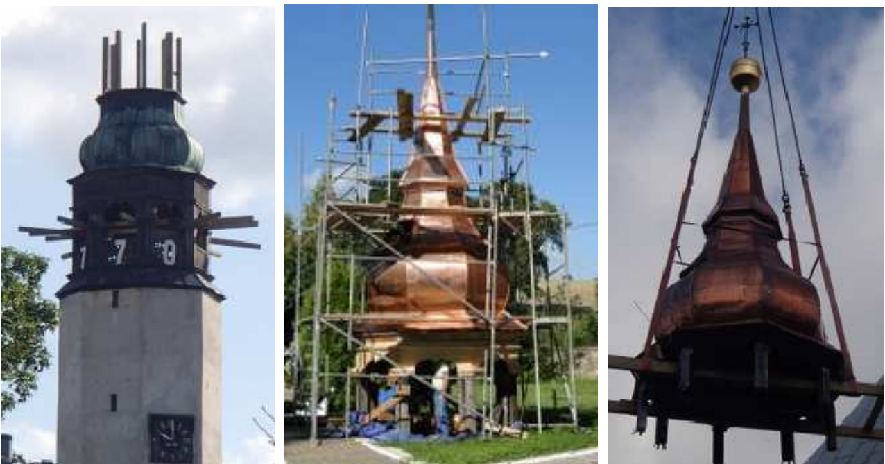
Figure 4: Removed upper dome for repair works (left) Repair of the upper dome on ground level (centre) Lifting repaired upper dome (right)
