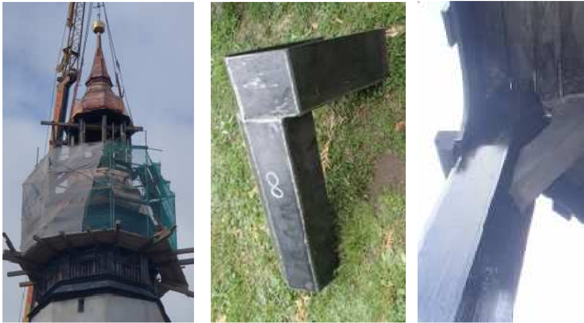
Figure 4: Repair of the upper dome on ground level (left) Connector for fixing upper dome (centre) After fixing (left)
