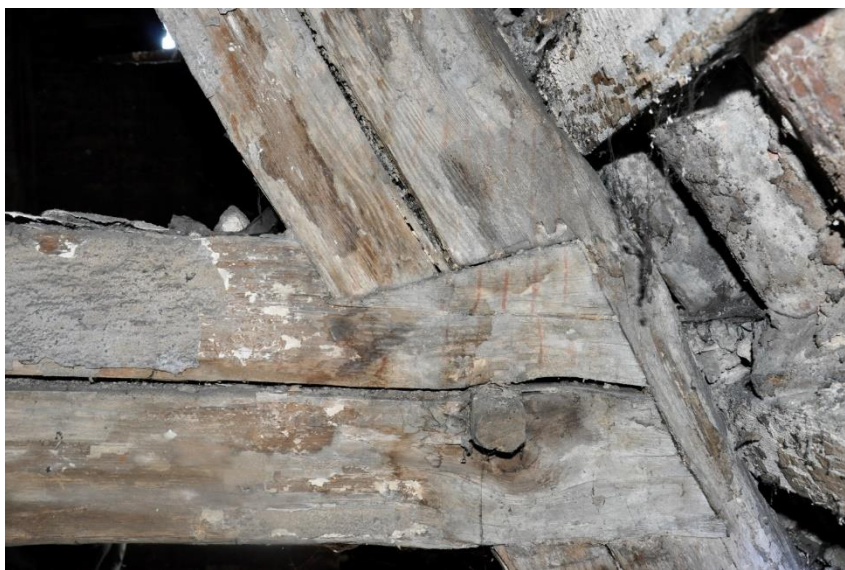
Fig. 3. Toruń, 6 Mostowa Street. Roof structure of building C. A carpenter's assembly mark made with a sanguine (Photo by U. Schaaf).
